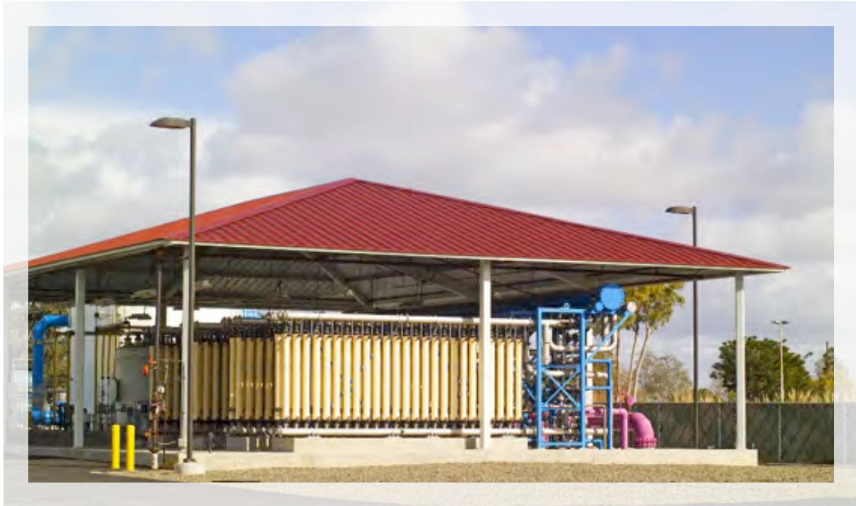
Microfiltration System at the LJV Facility
