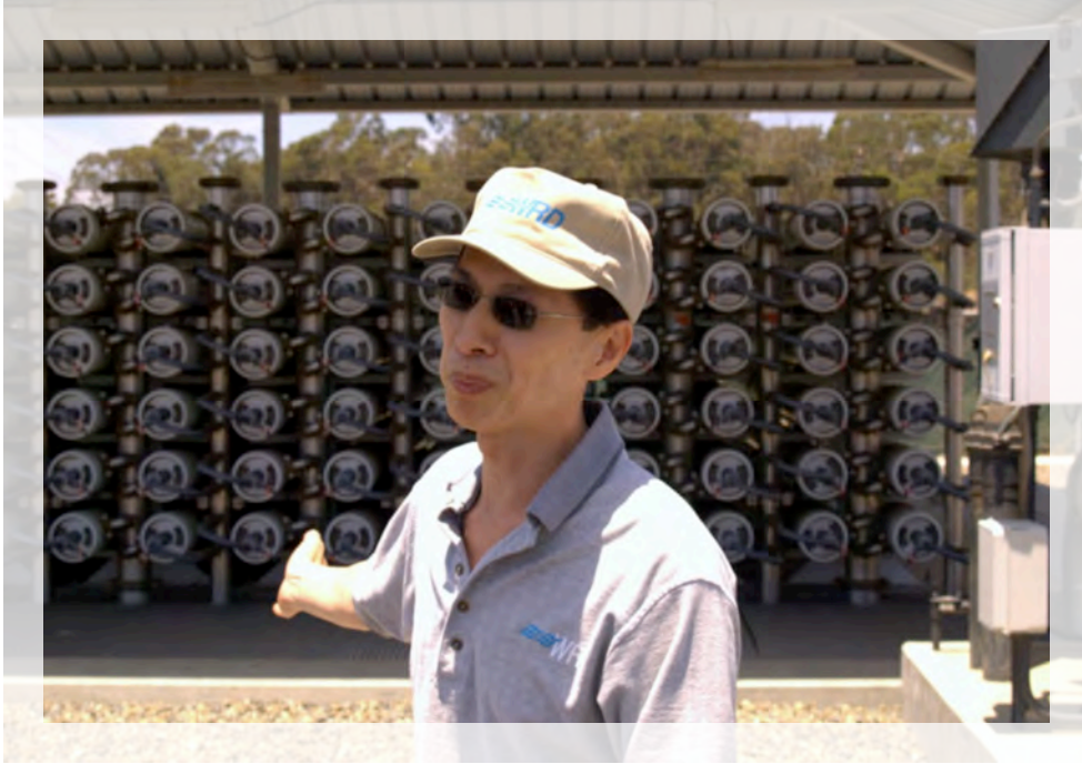
Reverse Osmosis System
