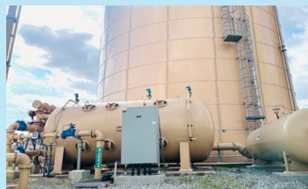
Maywood Mutual Water Company No. 2's Well 1 Treatment System
