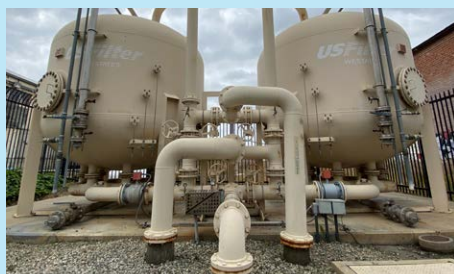
City of Commerce's Well #4-L Treatment System
