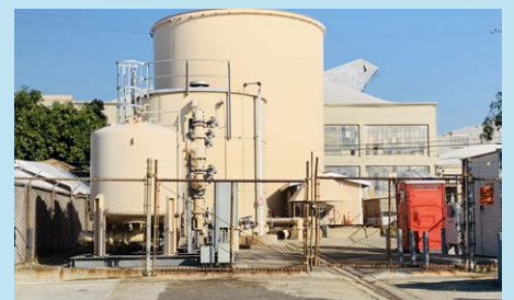
Maywood Mutual Water Company No. 2's Well 3 Treatment System
