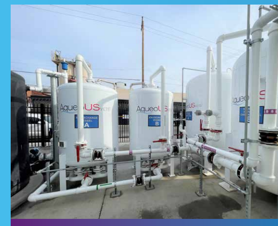
Groundwater treatment system to remove perchlorate in the Los Angeles Forebay
