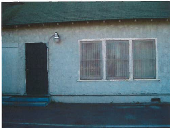
1913 building: View looking south at the east section of the north elevation
