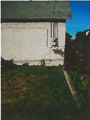
1913 building: View looking north at the east section of the south elevation; in the foreground are the foundation remnants of the rest of the building that had been demolished
