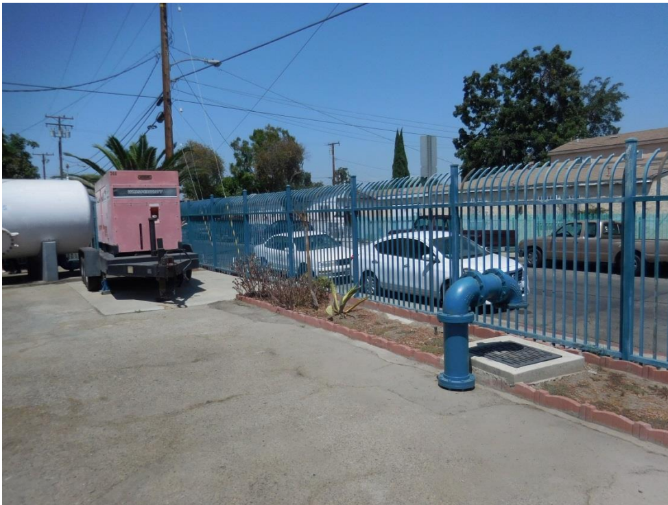
Photograph 2. View of backup generator facing north.
