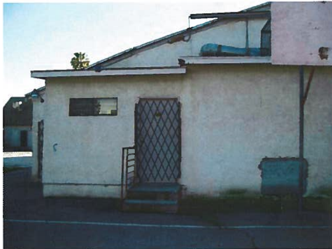
1947 building: View looking south at the east section of the north elevation
