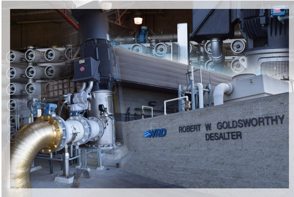
Robert W. Goldsworthy Desalter in Torrance, California
