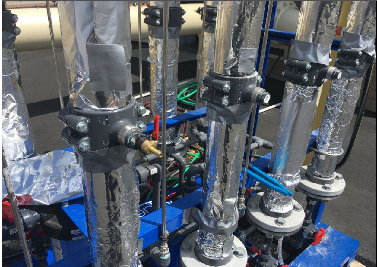
June 30, 2020, Midpoint sample ports were installed. Note that foil was added to the top of the columns and flowmeters on June 23 so there was no water or media exposed to sunlight.
